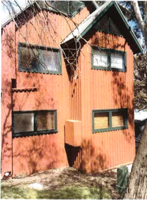
Figure 8 Western elevation displaying the Electrical Switchboard.
